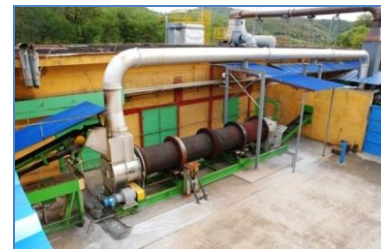
The EWI incinerator
